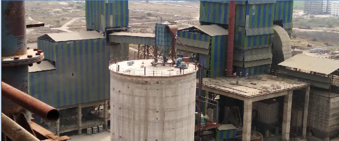
Bag Filters at Flyash silo Top
