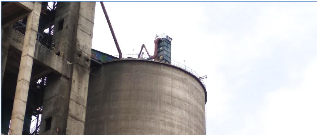
Bag Filters at Blending silo Top
