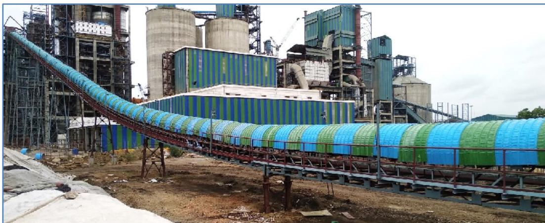
Closed Coal Conveying System
