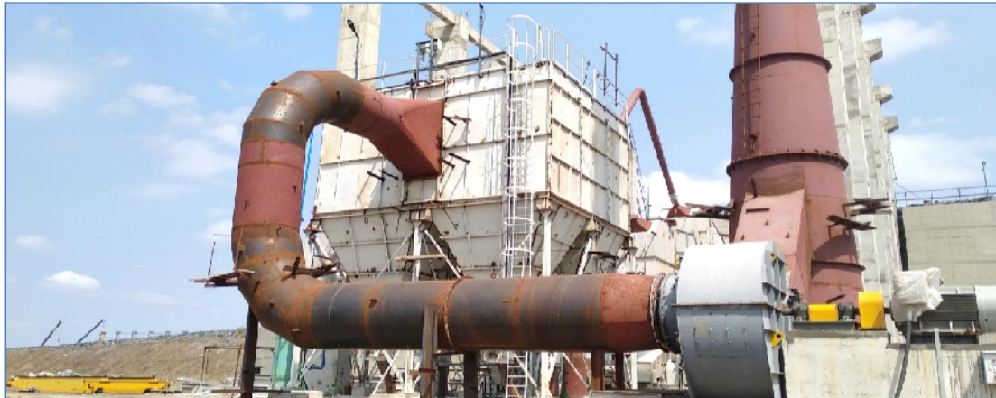
Bag Filter at Limestone Crusher
